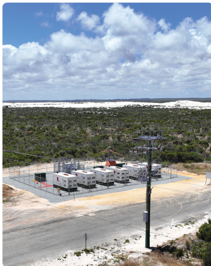
Figure 5: Lancelin HVIU and Emergency Response Generator facility
